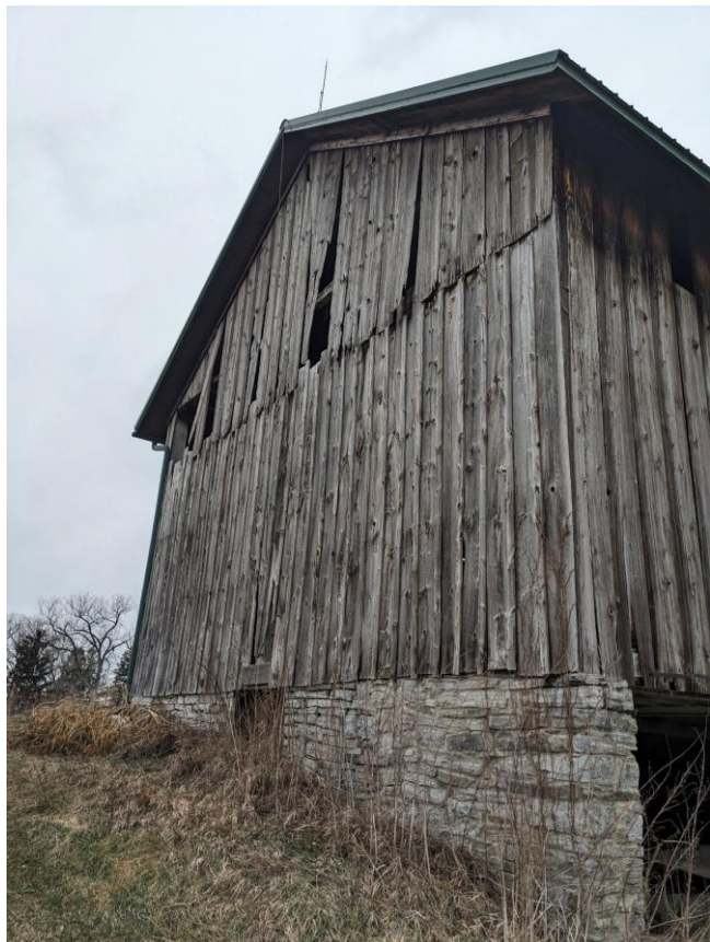
Big Barn - exterior wall and stone foundation; deteriorated siding is visible.
