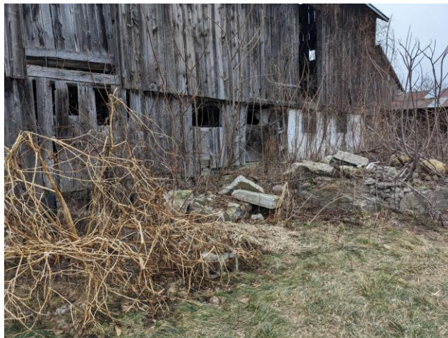
Big Barn - exterior condition near foundation; vegetation/debris and deteriorated building envelope are visible.
